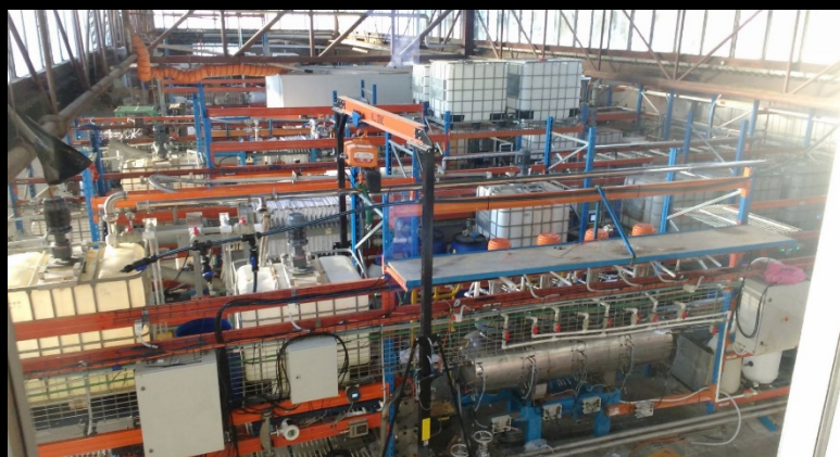
Perth demonstration HPAL plant
