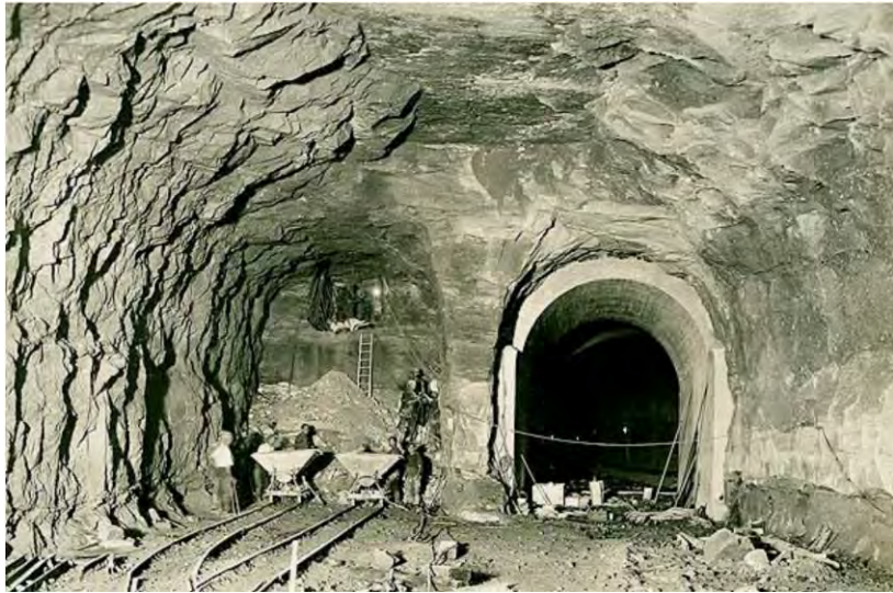
Junction of two 5 m tunnels and 11 m cavern. Bank St, North Sydney, 1925
