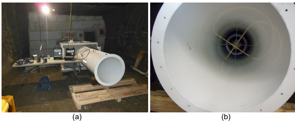
FIG 2 – Ventilation system controls (a) a two-stage fan and (b) a VOLU-probe.
