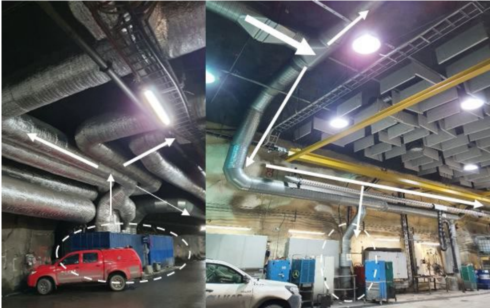
FIG 2 – Local area cooling on level 1250 for workshops, offices and restaurant (left, HEX containers circled), cooled air distribution in workshop (right, circled).
