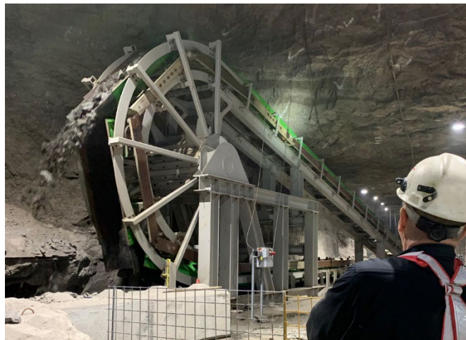
FIG 2 – A Railveyor underground discharge loop (source: https://www.railveyor.com/ ).
