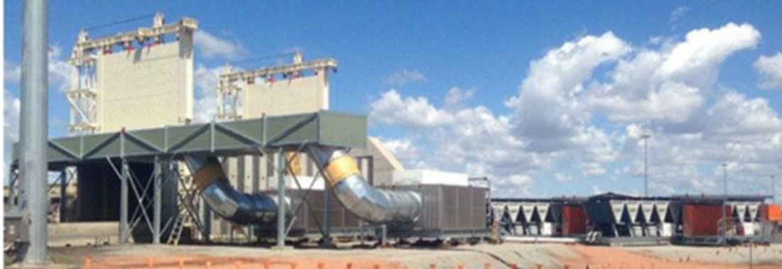
FIG 13 – Air-cooled refrigeration plant with BAC coils and air cooled chillers in the background.
