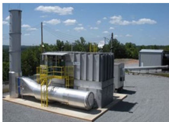
FIG 3 – First VAMOX® demo unit of 51 000 m 3 /hr capacity (2009).
