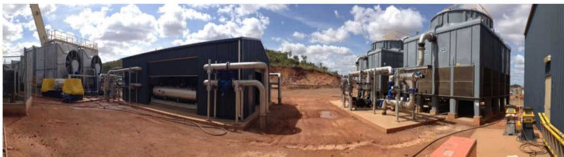
FIG 12 – Water-cooled refrigeration plant (permanent).
