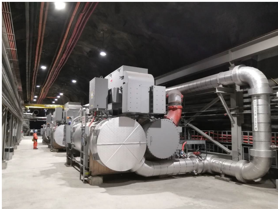
FIG 5 – View of complete plant room including insulated evaporator water piping.
