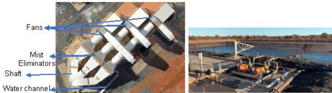
FIG 5 – VR6 mist eliminator and water sump: (a) VR6 fans and mist eliminator; (b) VR6 water dam.
