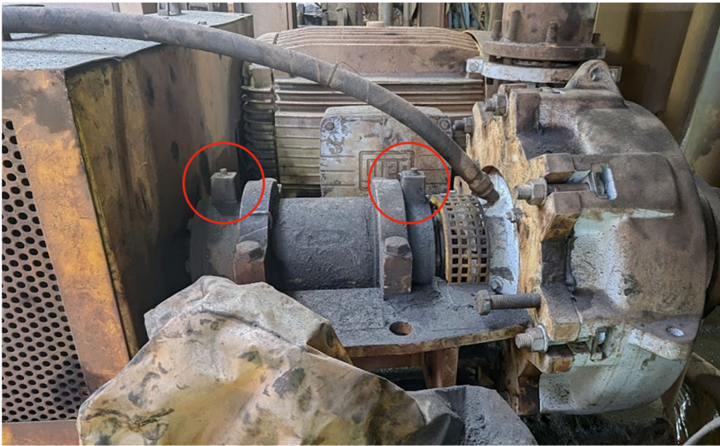
FIG 2 – Wireless sensors installed on slurry pump in red circles.
