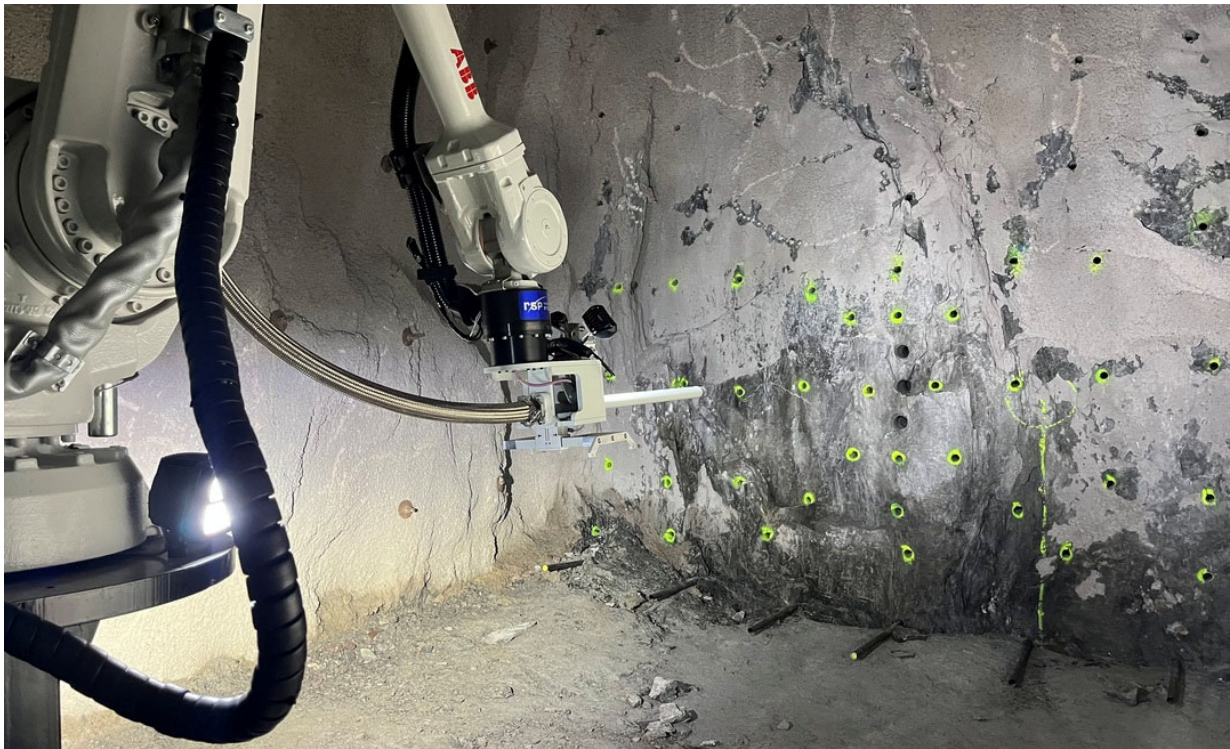
FIG 4 – Robot arm detecting the position of the drilled holes and then does the charging (image courtesy of ABB).
