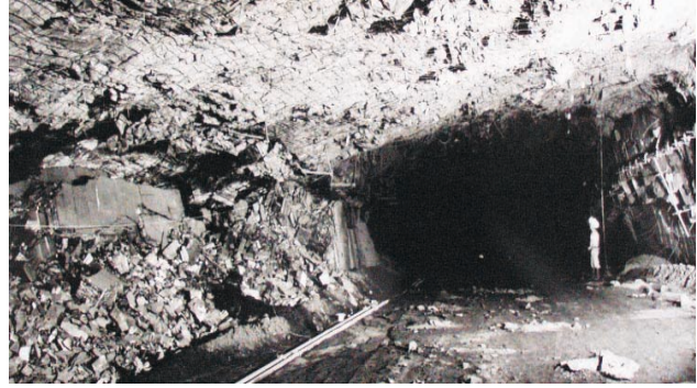
FIG 6 - A large stress-related footwall buckling failure.
